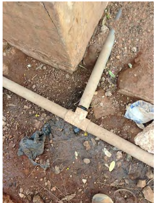
Figure 4-16: Broken distribution pipe (Photo: Deborah Vacs Renwick)
